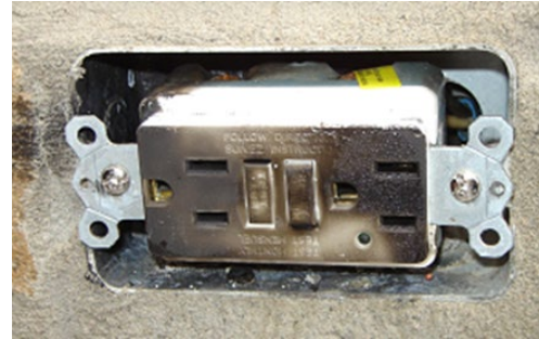
Although the GFCI tripped, the branch circuit conductors remained energized
