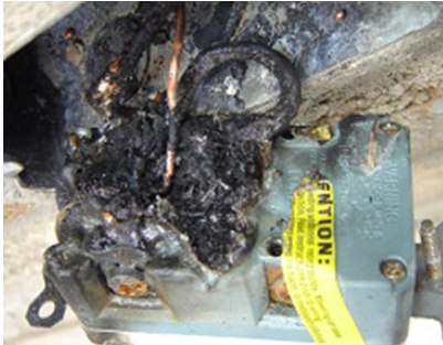
Moisture intrusion damaged the branch circuit conductors inside the receptacle box
