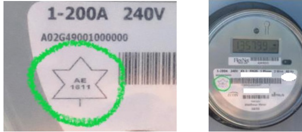
Photo B2 – Socket sub meter
