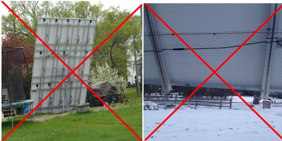
Photo B5 – examples of non-compliant installation
