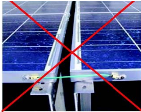
Photo B1 – Unacceptable bonding conductor connection
