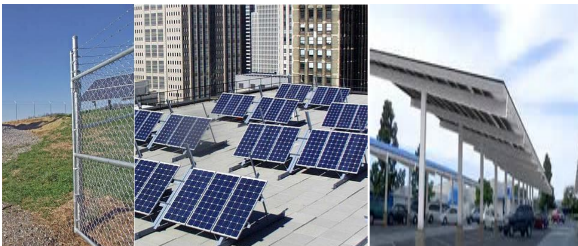
Photo B1 – Examples of PV source and output circuits considered not accessible to the public
