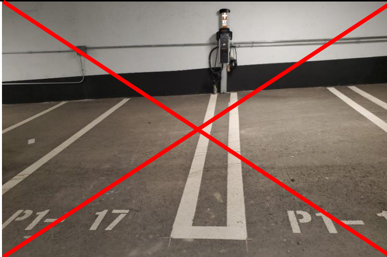
Photo B6 – Example of protection by location not acceptable.
